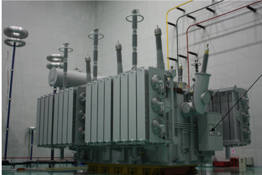
Example: JSHP 345KV transformer (supplying 10% of the New York City load)
